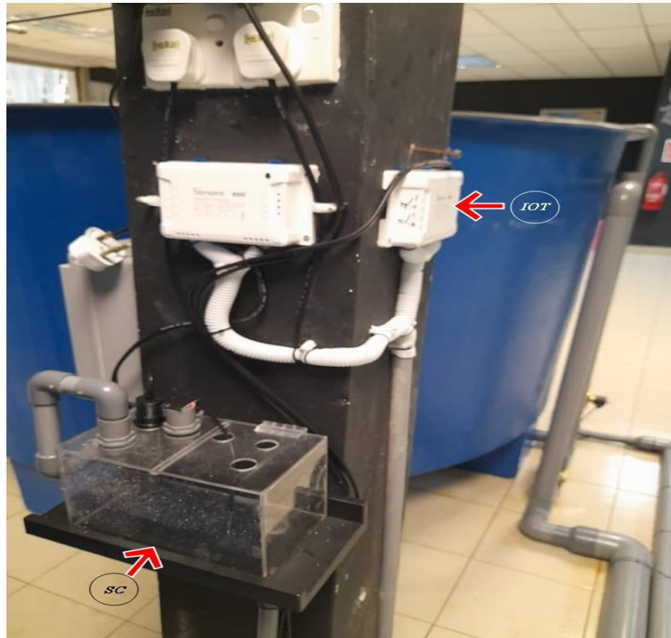
Figure 4.4: The production unit showing the water sampling chamber with sensors and the IoT of IMTAS
